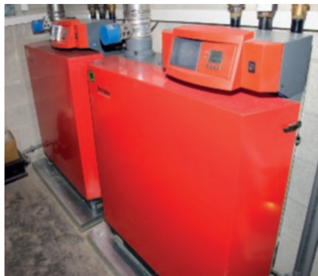
Remeha Gas 210 ECO PRO (16 tot 200 kW) Project Cadix Factory Antwerpen
